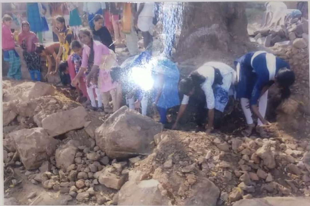
N.S.S. volunteers working to construct Aralikatte (public gathering place) at maratageri adopted village
