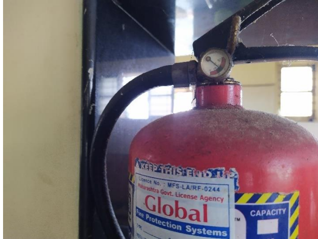
Figure 15 - Ready access to fire extinguisher.
